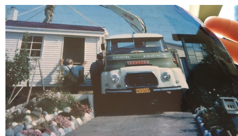
From Left: Ted, McDowell, Charlie McDowell and Bob McDowell working the Hiab controls.
